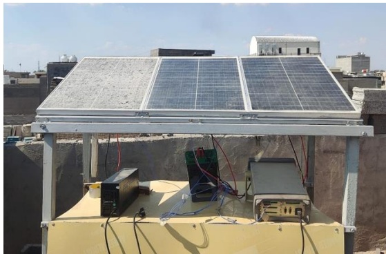
Figure 3. Effect of dust accumulation on PV modules on 30/4/2026 showing the reference PV module (left), \text{TiO}_2 -coated PV module (center), and \text{SiO}_2 -coated PV module (right) under real operating conditions
