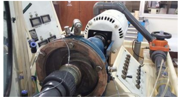
Figure 3. Accelerometers installed on the pump casing.
