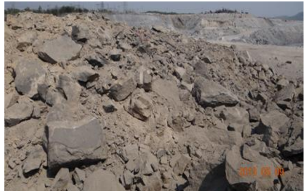
Figure 27. Fragmentation obtained using the pilot holes and pocket charges at the 1 st Bench, Matin-Di area.
